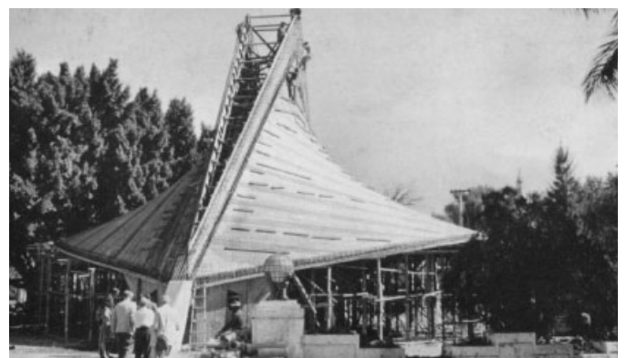
Felix Candela, Hyperbolic paraboloid roof surface, Mexico, under construction The warped, double-curved surface is constructed by a series of straight lines that allow the use of straight timber planks as formwork.
