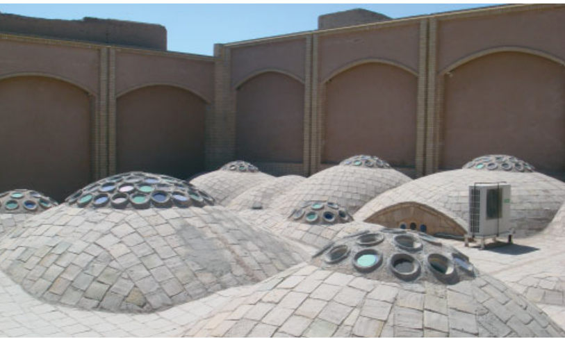
The roof of this historic bathhouse in Yazd, Iran, shows the typical domed surface used for self-shading. The air conditioning, which was installed when the building was converted into a coffee house, required the closing of the air vents of the domes, which now only serve to bring light into the interior.
